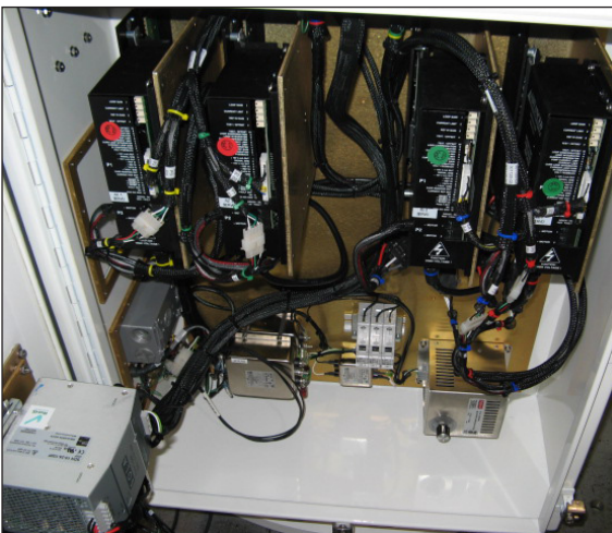
The Pedestal Interface Unit (PIU) contains all of the pedestal electronics.
